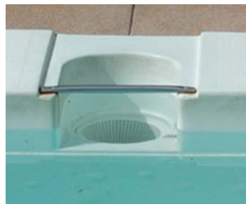
Dangerous skimmer box
